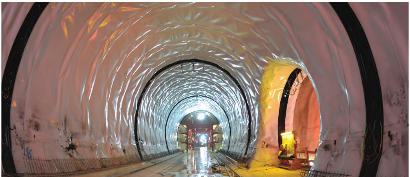
Waterproofing in the Alabstieg Tunnel, new Wendlingen–Ulm rail route (Source: Deutsche Bahn AG)
