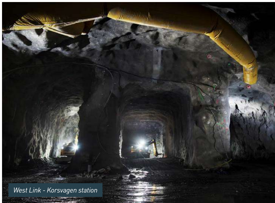
Extensions of the subway in Stockholm
