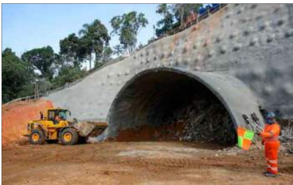
Contorno Viário de Florianópolis: Tunnel 1 begins to be excavated in Palhoça (Photo: Arteris, Disclosure)
