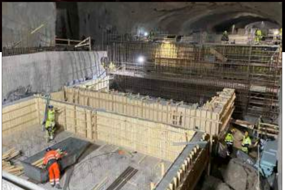
Tampere Region Central Wastewater Treatment Plant Sulkavuori
