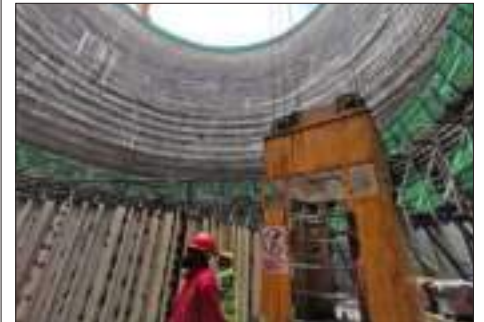
Suki Kinari Hydropower Project
