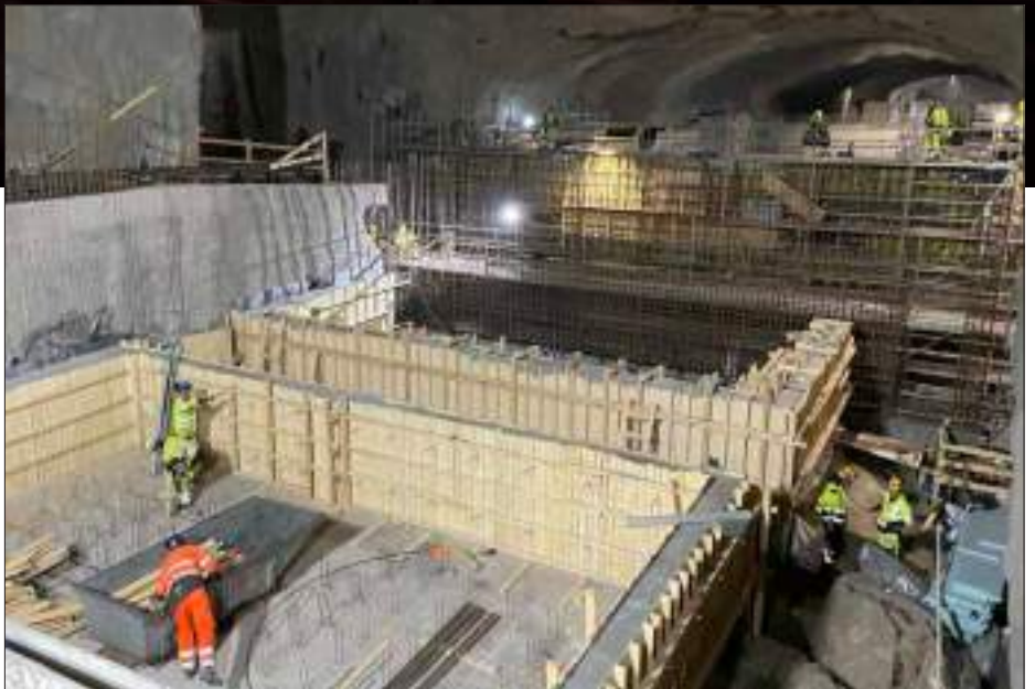
Tampere Region Central Wastewater Treatment Plant Sulkavuori
