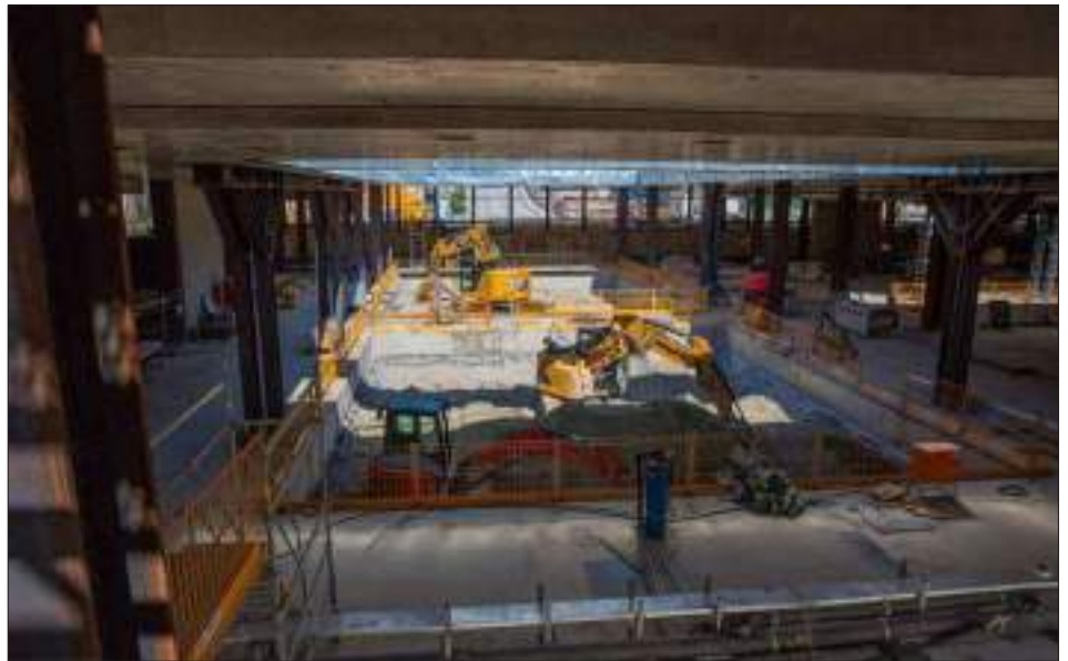
Munich's 2nd Core S-Bahn – Excavation work on level –2 at the Central Main Station construction site (Source: DB InfraGo AG/panterra.tv)
