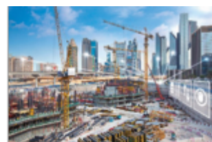
Deformation monitoring system
