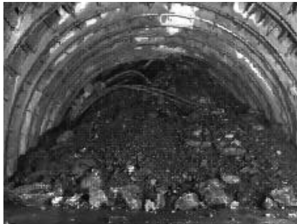
Collapse in a road tunnel in glossy schists
